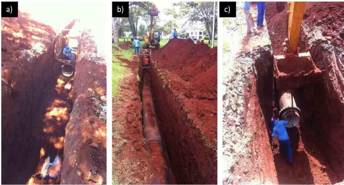
a) and b) Employees inside the containment shield; c) Employees without the use of containment shielding.
