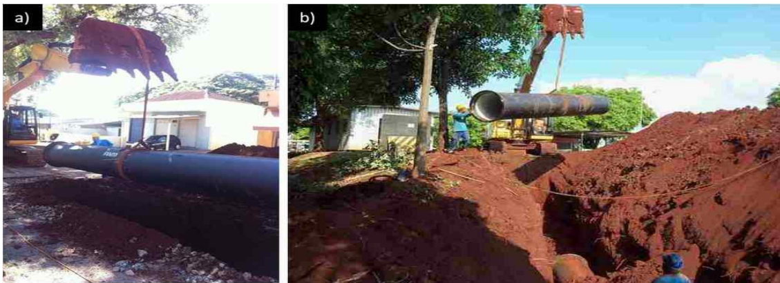
a) Piping with lifting strap; b) Employee guiding piping for laying in ditch.
